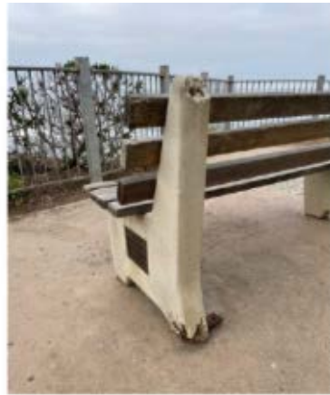
The popular Forward St. ocean overlook bench (left) was noted as needing replacement for many years. Following interim repairs of deteriorated wooden slats over the years, it was time to address exposed rebar, deteriorated concrete, failing bolts and screws, rotted wooden slats, and other damage.
